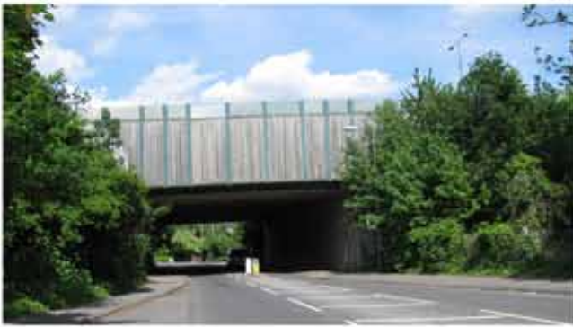
The M25 bridges over Woodham Lane, visually screened from the public realm
