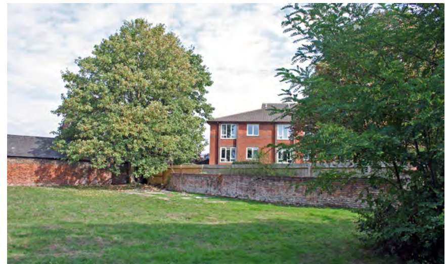
Dilapidated stretch of boundary wall in St John the Baptist's churchyard
