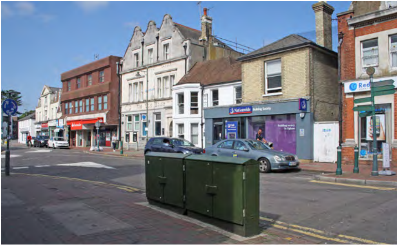
Example of pair of broadband cabinets on the High Street
