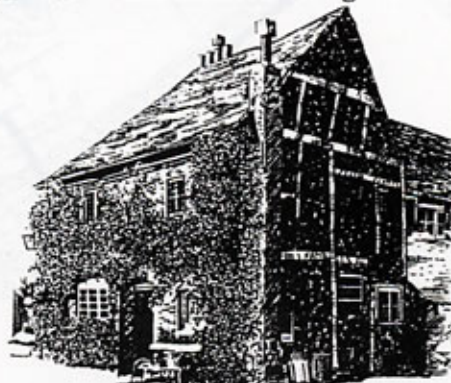
The rear elevation of Thorpe Farm, Village Road, shows the timber framing of the 17th century core of the building. This is hidden behind later remodelling on other elevations.
